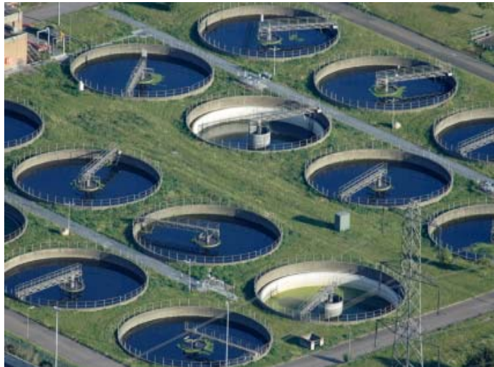
Figure 3: Sedimentation tanks, such as those shown above, are used to settle the sludge and remove oils and fats in sewage. This step can remove a good portion of the biological oxygen demand from the sewage, a key step before progressing with the treatments and eventually releasing into the ground or body of water.
